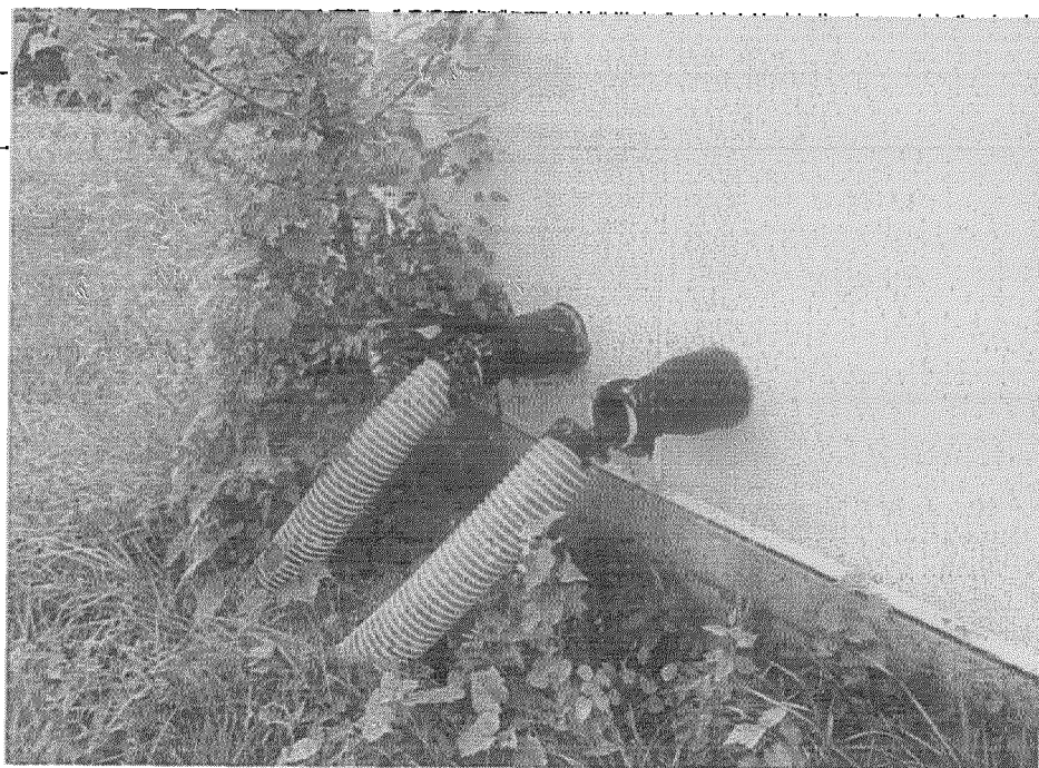
Bureau Id: 1770200010 Photo No.: 6 Photo Date: 8/4/2023 Photo Time: 10:12:54 AM Direction: SE Taken By: Rebecca DeMay
